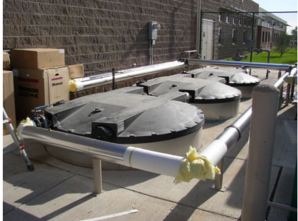
Ice storage for building cooling
